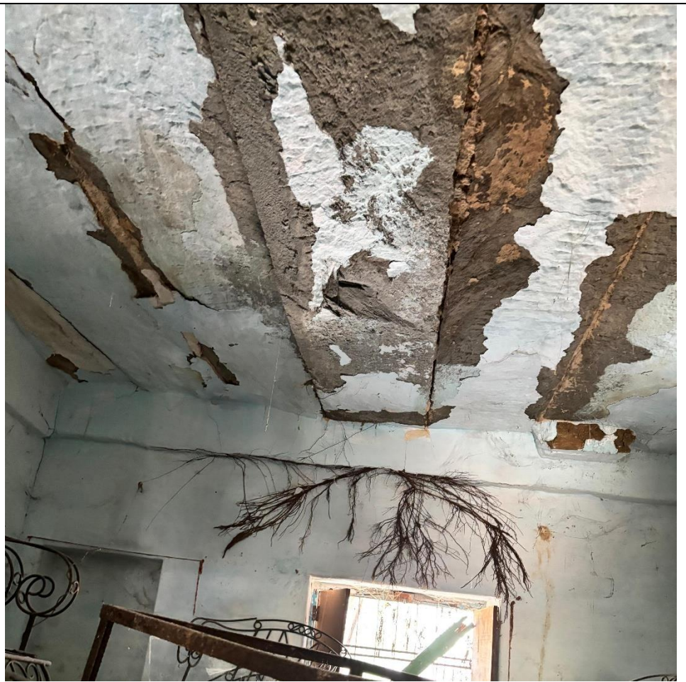
Roots of the vegetational growth inside the structure
