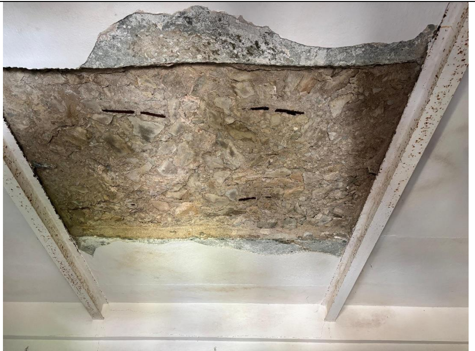
Portion of Lime concrete sank in inside the monument
