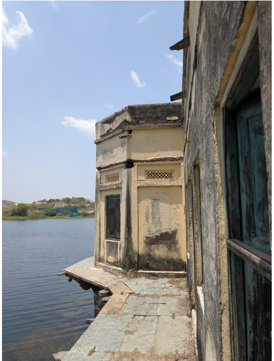
Lost MS railing and broken floor tile.
