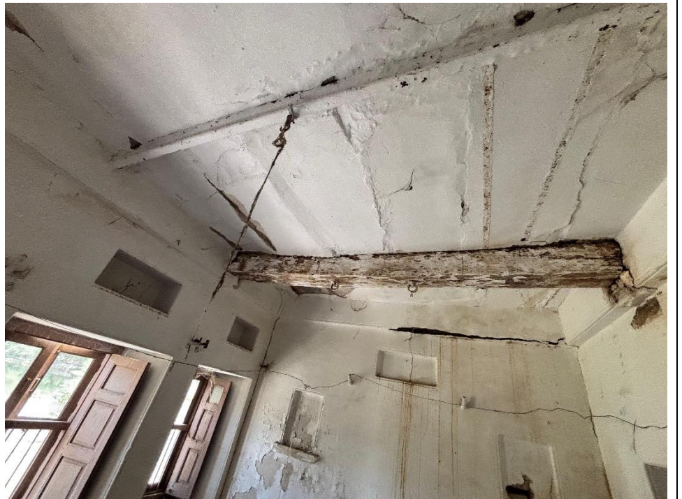
Wooden beam and sunken roof gone out of plum.
