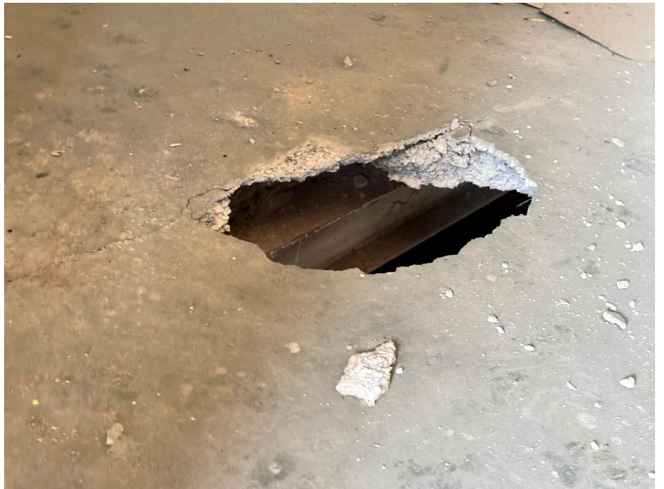
Caved in roof inside the monument.
