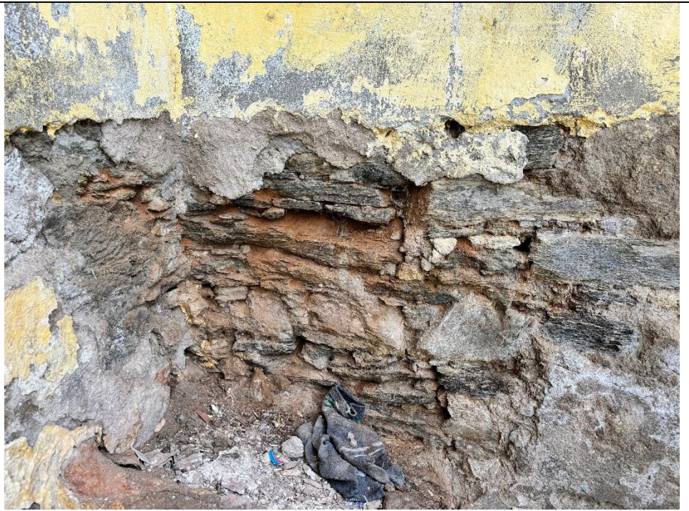
Lost / extensively damaged masonry
