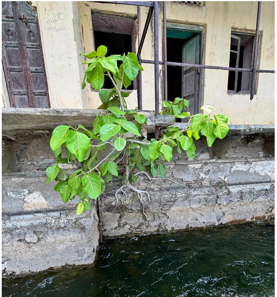
Large vegetational growth on the water front side wall
