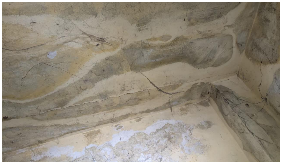
Cracks in roof.
