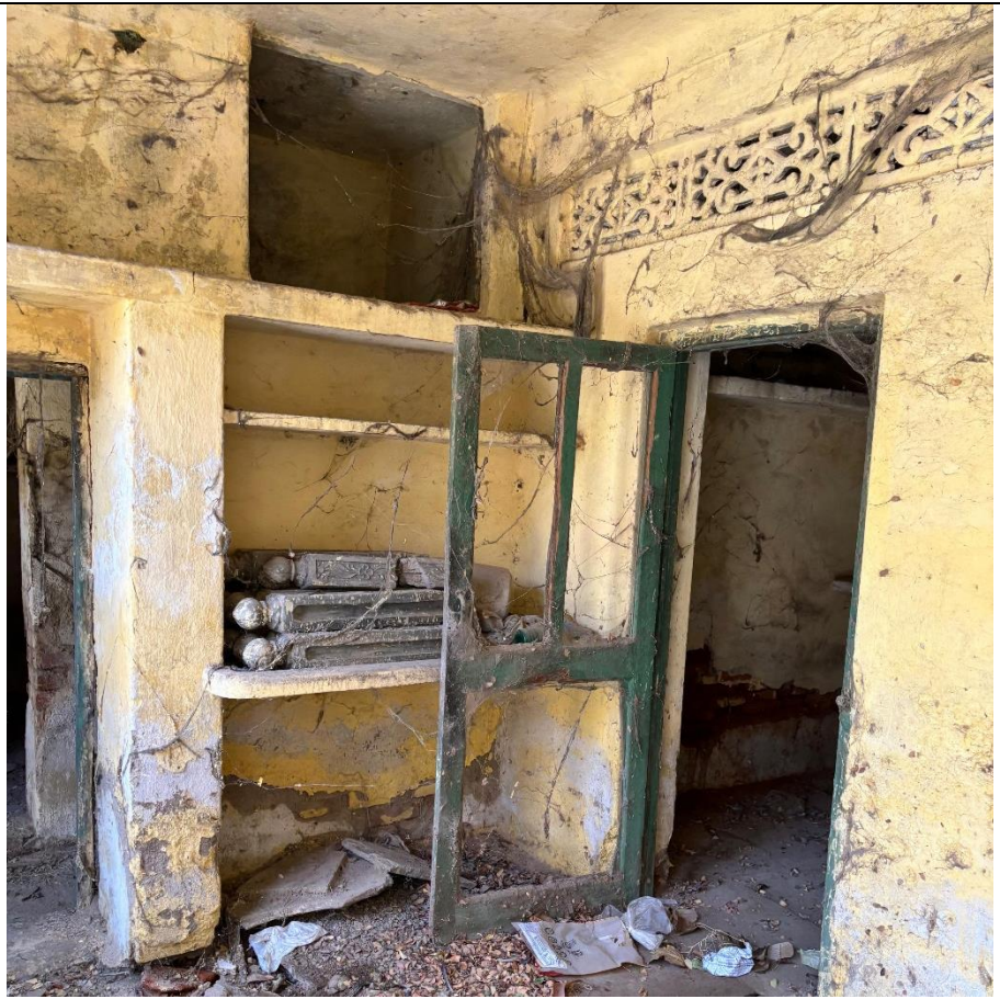
Damaged Doors and Windows
