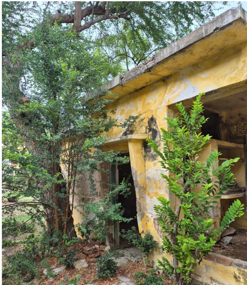
Tree causing damage to the walls
