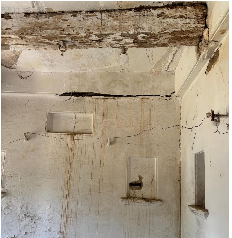
Large Cracks on beam causing water seepage
