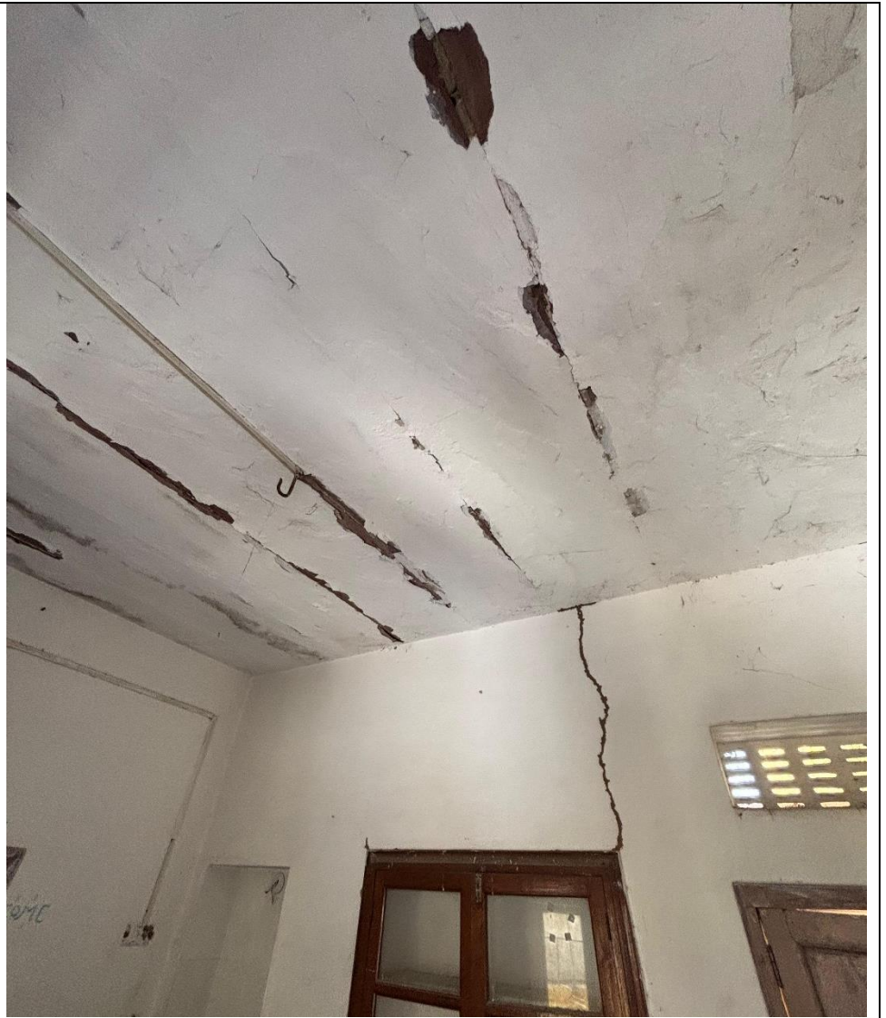
Termite and major roof cracks.
